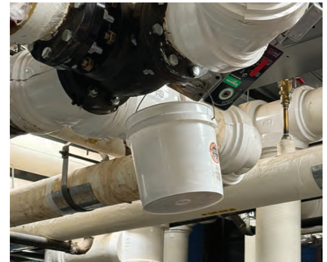
Buckets used to catch leaking pipes are just one of the many maintenance repairs that would be made if the bond issue passes
