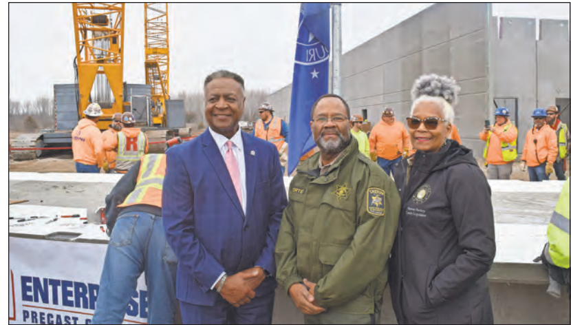
(L-R) County Executive Frank White Jr., Sheriff Darryl Forté, and legislator Venessa Huskey stand beside the final beam before its placement.
